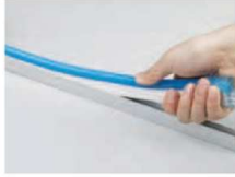
Linear Installation 1. Aluminum Channel FN113 2. Apply an adhesive silicone between the channel base on fixture housing to prevent slippage and stretching over time
